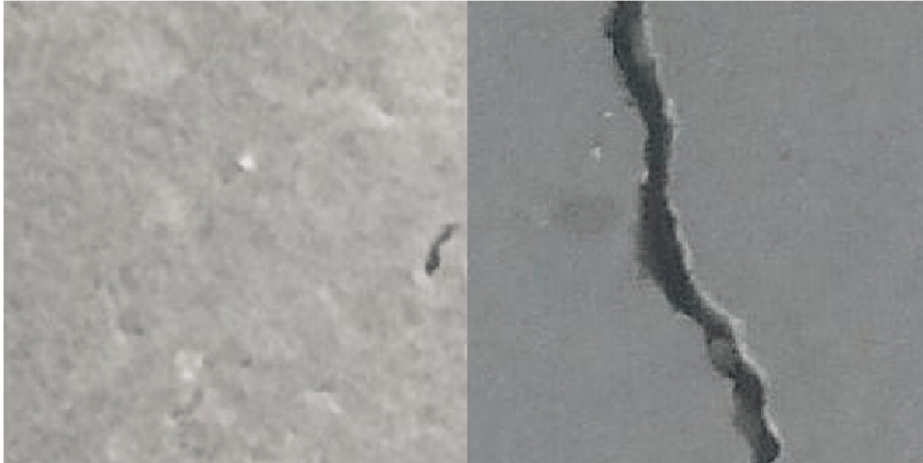
Road Images Without (Left) and With (Right) Crack Anomalies
